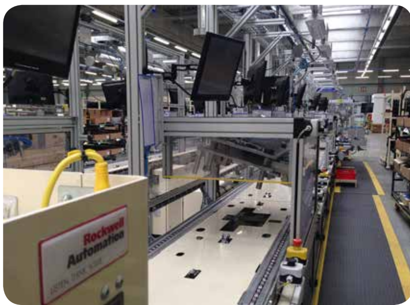
PHA Czech s.r.o. tasked the Rockwell Automation Global Solutions team in the Czech Republic to develop a complete control solution for a front/rear, left/right turnkey door module assembly line and end-of-line (EOL) test stations
